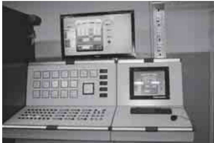
Fig. 3. Operator station EMOS
