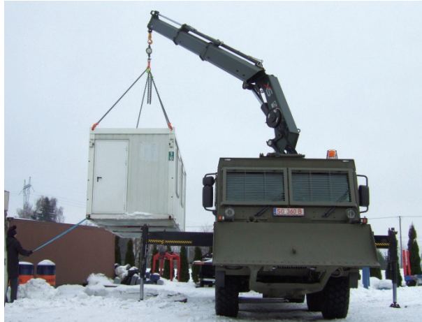
Fig. 16. View of the container sized 1C lifted by the crane from the ground
