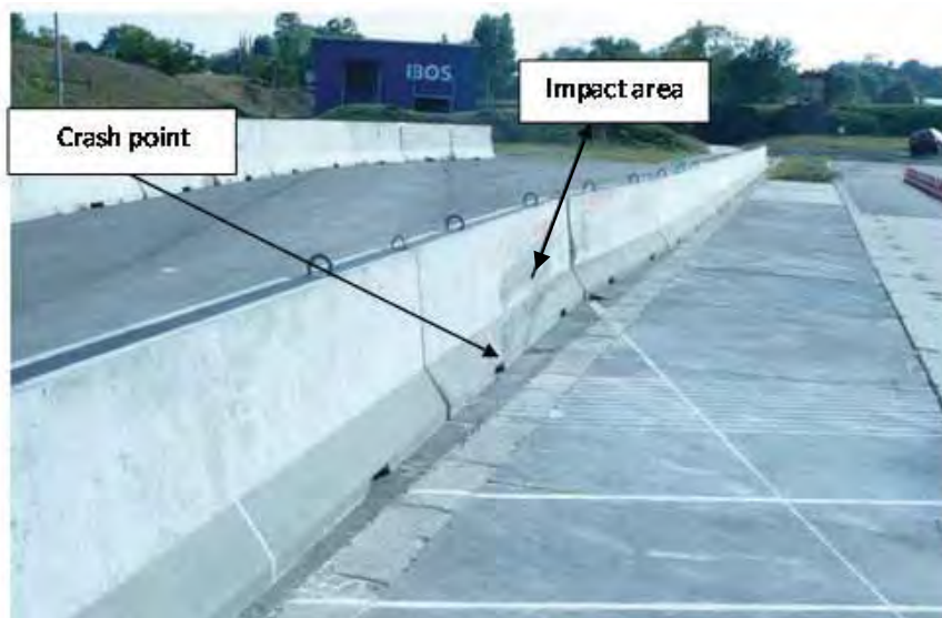
Fig. 5. The prototype concrete protective barrier after the crash test – visible crash point, impact area and final barrier deformation
