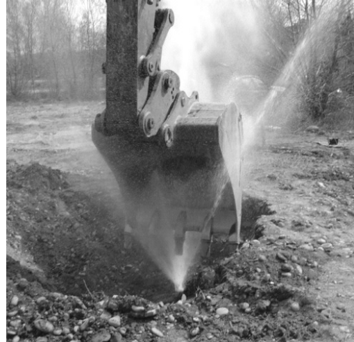
Fig. 2. Consequences of inattentive diggings [3].
