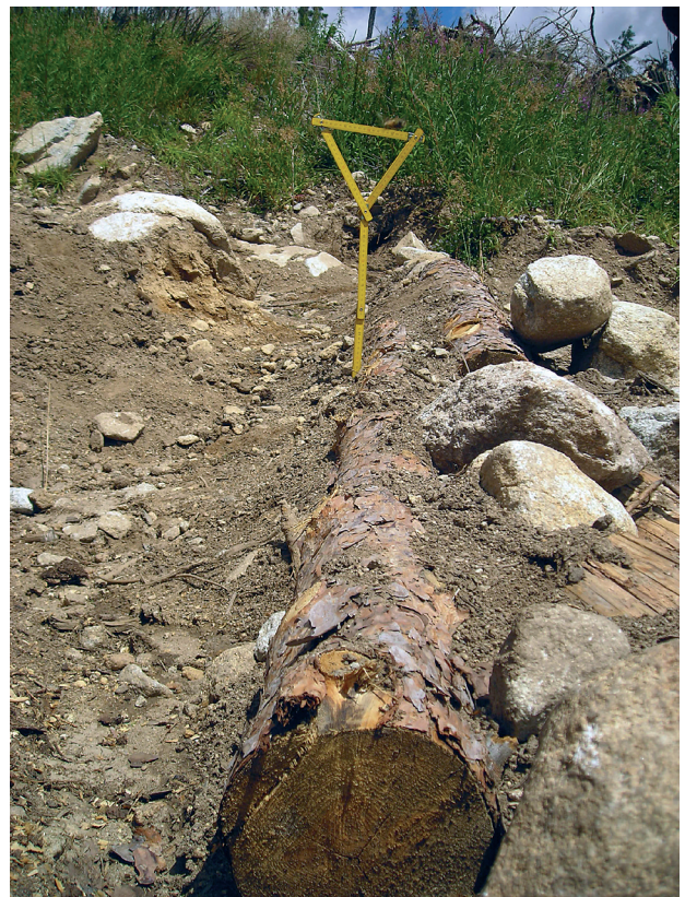
Fig. 7. One of anti-erosion steps on a cart road in Nová Polanka
