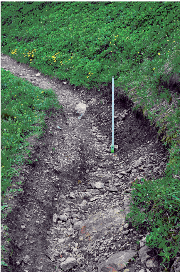
Fig. 3. Fresh erosion furrow after intensive rain precipitation on hiking trails in the Zadné Meřodoly Valley. Photo: J. Hreško, June, 16th, 2008
