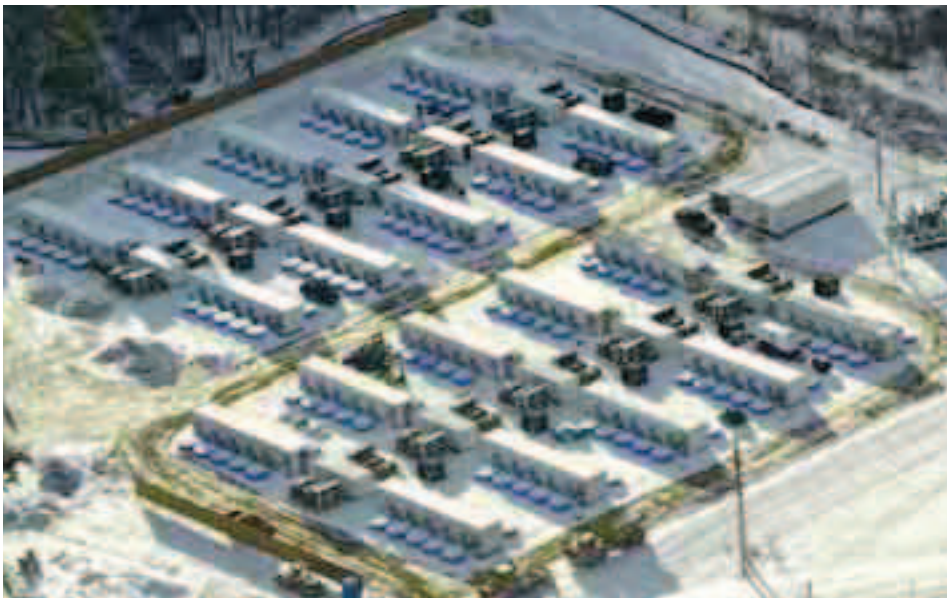
Fig. 8. A 20 MW plant constructed in Stephentown based on flywheels (NY, USA) [8]
