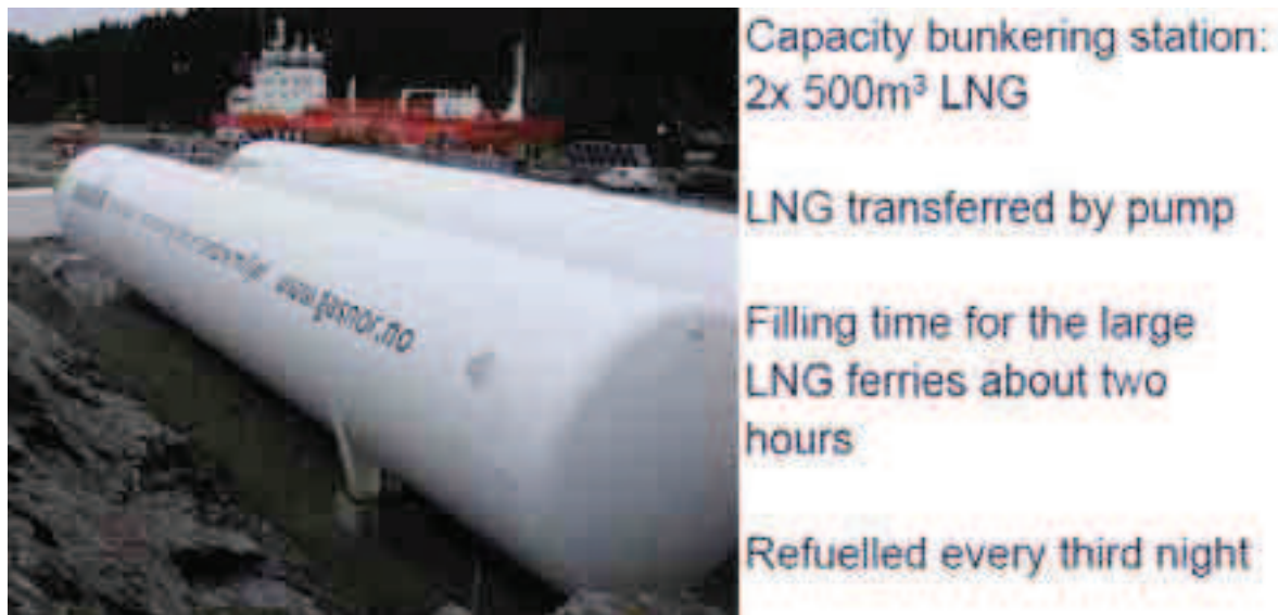
Fig. 5. LNG bunkering station at ferry berth for m/v Bergensfjord [10]
