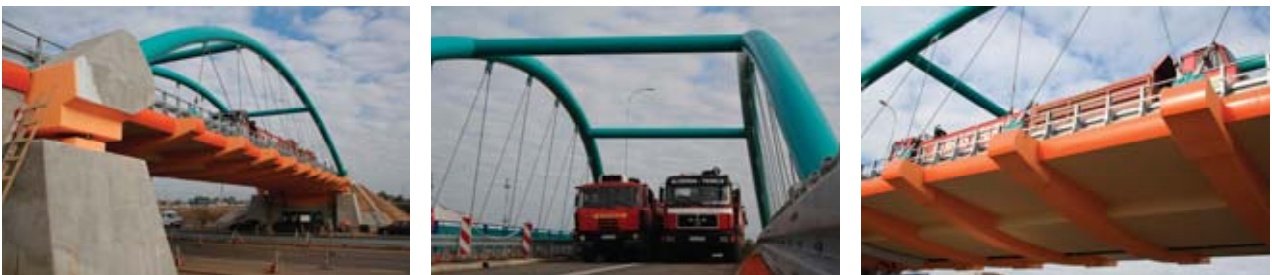
Fig. 11. Construction of the arch span of the viaduct in Nowy Dwor Gdański
