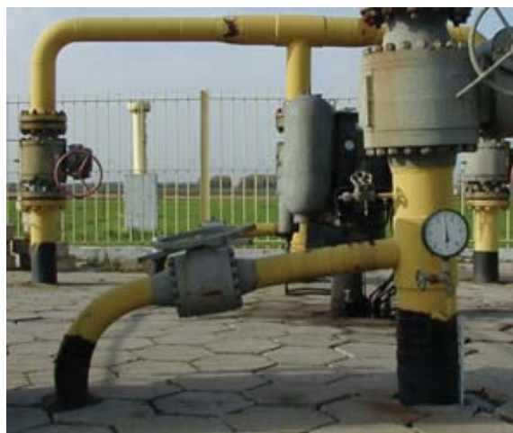
Fig. 2. The block valve station subjected to numerical analysis
