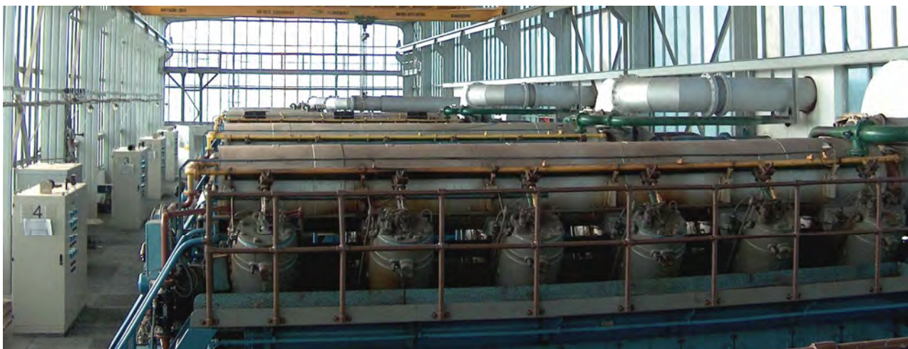
Fig. 1. An engine-compressor installed in one of the gas transmission stations
