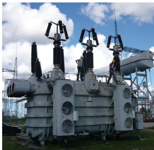
Rys. 1. Transformator RTdxP 230/110/15,75 kV, 160 MVA użyty do badań Fig. 1. RTdxP 230/110/15,75 kV, 160 MVA transformer used for the experiment
