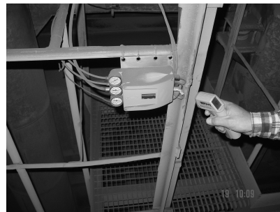
Fig. 1. High temperature (up to 75°C) and dusty environment significantly cut down the actuator lifetime applied in the boiler section of a power station. Snap was taken after two months of putting a new positioner for the operation
