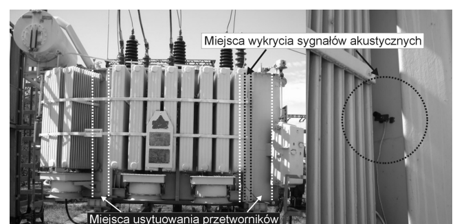
Rys. 1. Widok badanego transformatora Fig. 1. Overall view of the transformer under study
