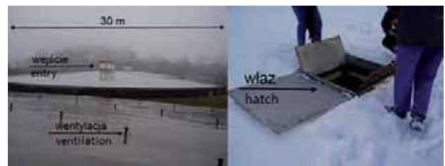
Fig. 2. Tanks for storing water – MPWiK Cracow
