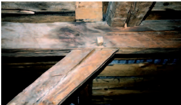
Fig. 1. View of the cracks in the angle brace, the purlin and the rafter
