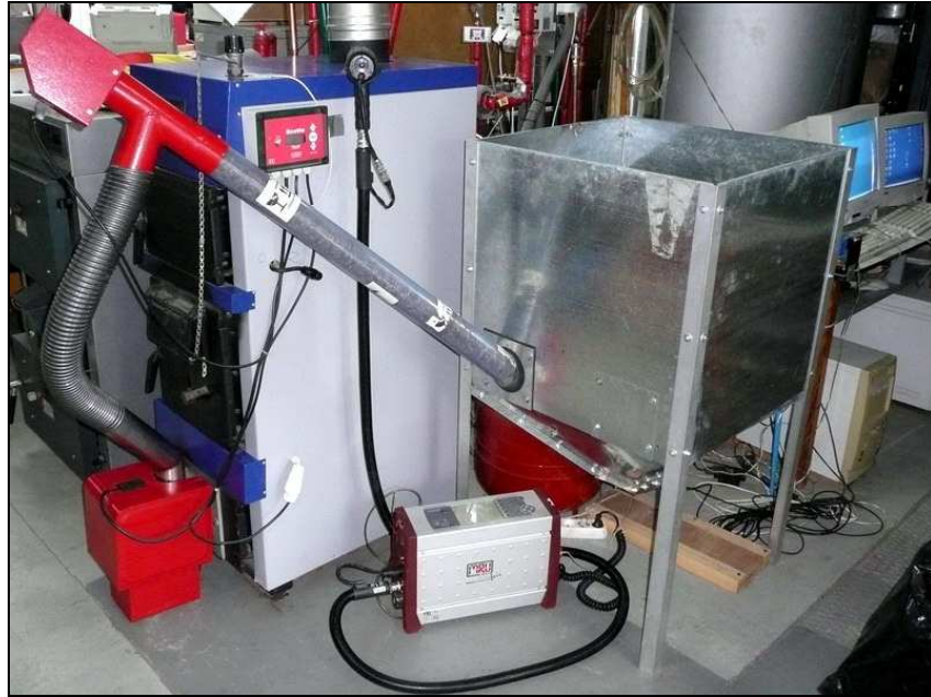
Fig.1. Heat station with two wood log boilers: with a heat output of 15 kW (with a pellet furnace) and 25 kW (with wood gasification)
