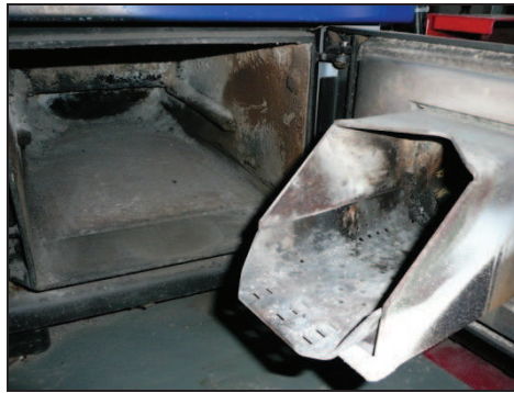
Fig. 2. Furnace view: fixed-speed screw pellets dispenser; air outlets
