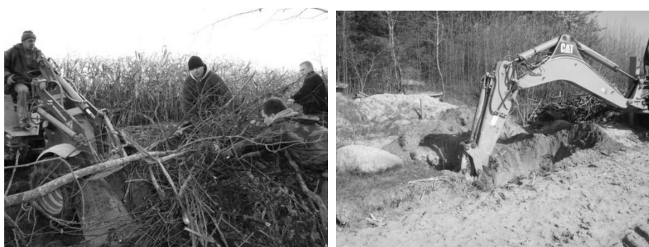
Rys. 7. Oczyszczanie terenu mogilnika. Praca koparki na terenie mogilnika Fig. 7. Refining of graveyard area. Excavator near graveyard
