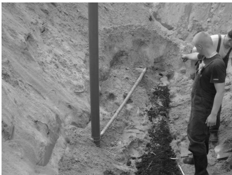
Rys. 10. Piezometr wraz z fragmentem bariery Fig. 10. Piezometer with drainage and part of compost barrier
