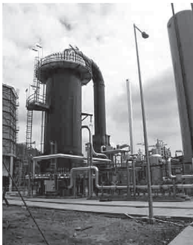
Photo 2. Hydrogen Production Plant reformer
