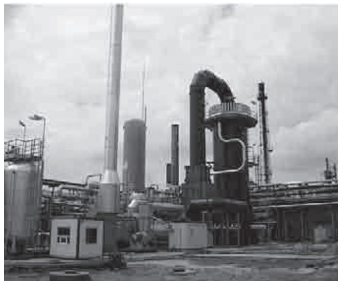
Photo 1. Hydrogen Production Plant. Capacity: 8,000 Nm 3 /h of H 2
