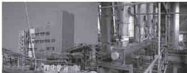
Photo 7. Assembly of instruments and devices according to the progress in constructing the installation building
