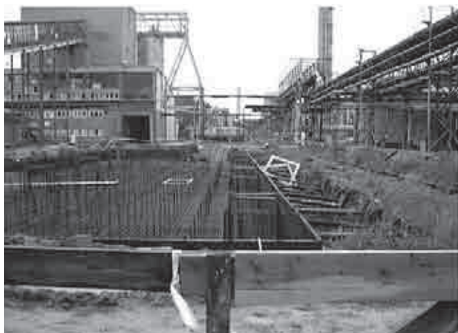
Photo 3. Building foundations for the main building and construction of a drum dryer
