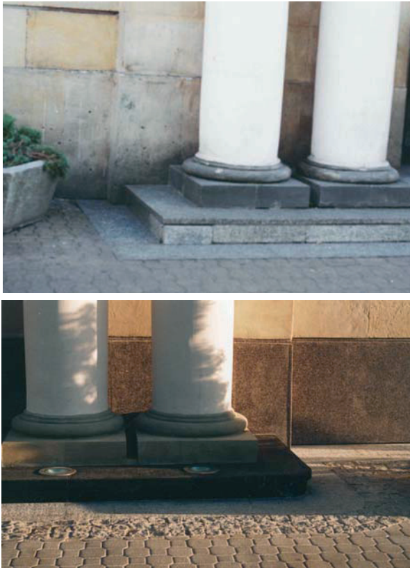
Photo 3. View of the pavement at the main entrance before and after renovation.
