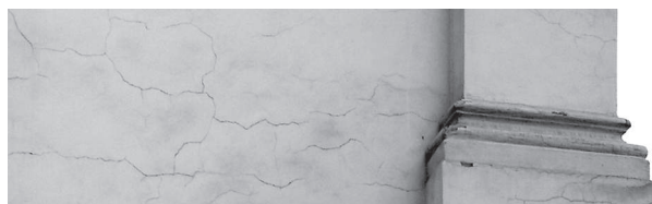
Fig. 12. Cracks in the chapel walls of the Holy Trinity Church
