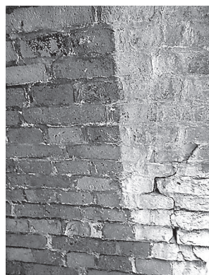
Fig. 15. Surface of bridge before cleaning
