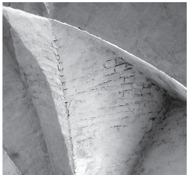
Fig. 5. Corrections in the direction of the courses carried out ad hoc by cutting bricks, indicate that the vault was constructed without formwork (D. Wendland)
