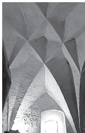
Fig. 2. “Cell Vault” in Trebsen (Germany), where the curves, surfaces and also the masonry textures could be surveyed and analyzed (D. Wendland)
