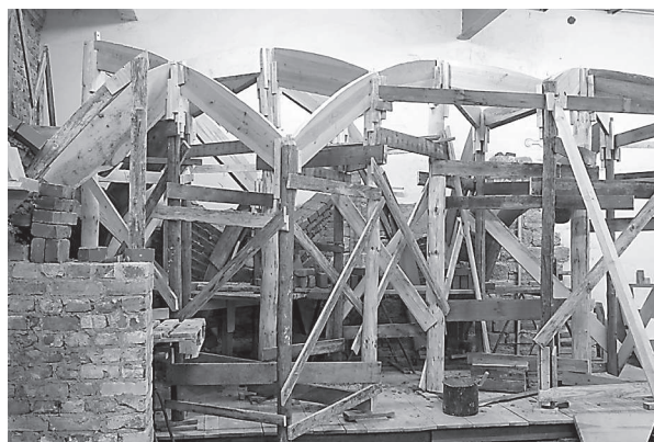
Fig. 15. Reconstruction of the centering used for building late Gothic “Cell Vaults”, developed from surveys in correlation with sources and the experience of the experimental reconstruction (D. Wendland)
