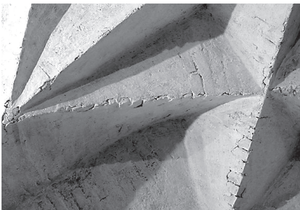
Fig. 9. Due to the continuity of the masonry texture, the courses are not arranged perpendicular to all groins, as usually assumed. Such observations lead us to understand the construction principles and rules applied by late Gothic masons (D. Wendland)
