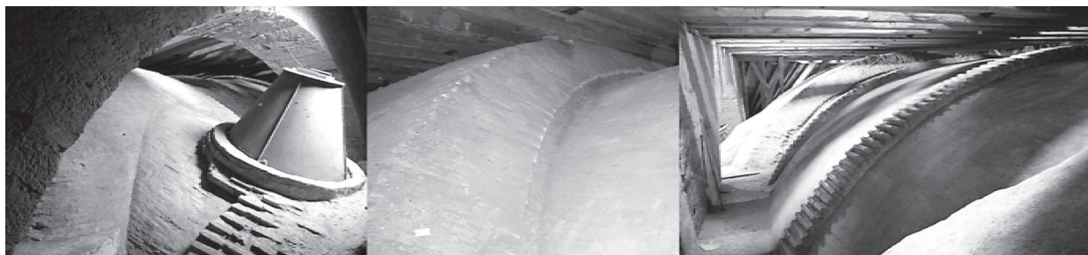
Fig. 4. Church at the Benedictine monastery of Banz. Brick masonry roof viewed from the extrados
