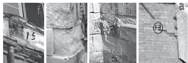
Fig. 26 Photos showing different deterioration aspects such as human intervention, back weathering, bio-deterioration and water penetration respectively.
