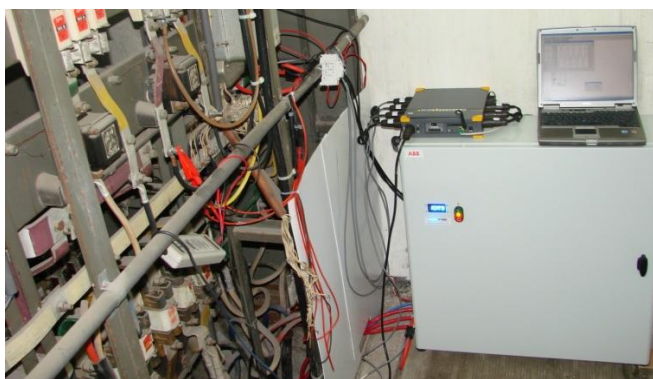
Fig. 3. The new capacitors bank connected to the LV busbars by the cell (bay) of switchgear in power supply station of factory.
