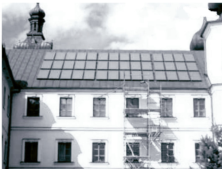
Fig. 1. South oriented solar collectors on a roof at the Cloister of Redemptorists, Tuchow, Poland
