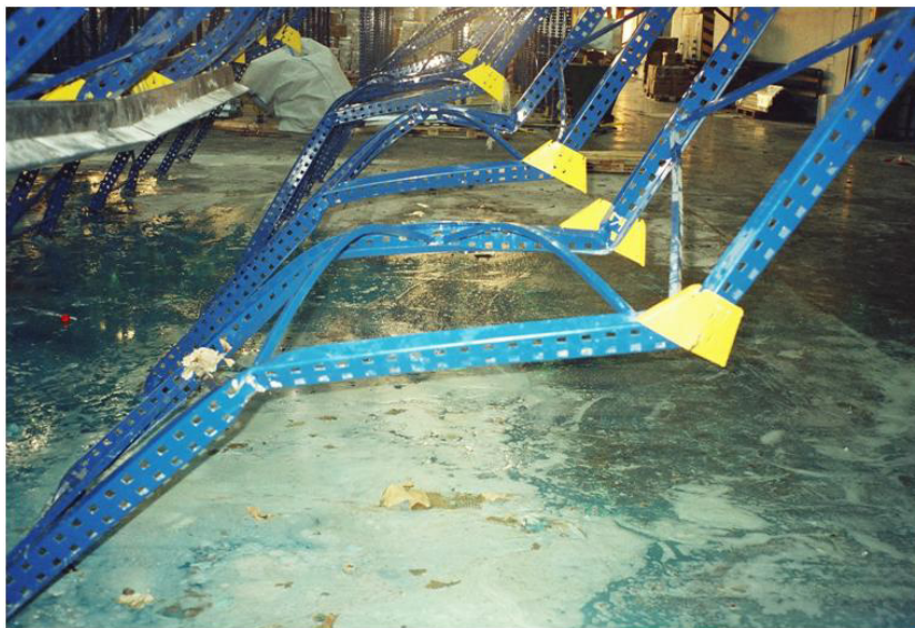
Fig. 2. Destroyed multi-level storing frame after collapsing
