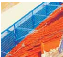
Photo 6. Metal-guard side protection placed on the edge of a roof
