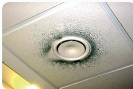
Fot. 1. Anemostat nawiewny zanieczyszczony cząstkami aerozolu ziarnistego i bioaerozoli Photo 1. Supply air diffuser contaminated by aerosol particle matter and bioaerosols
