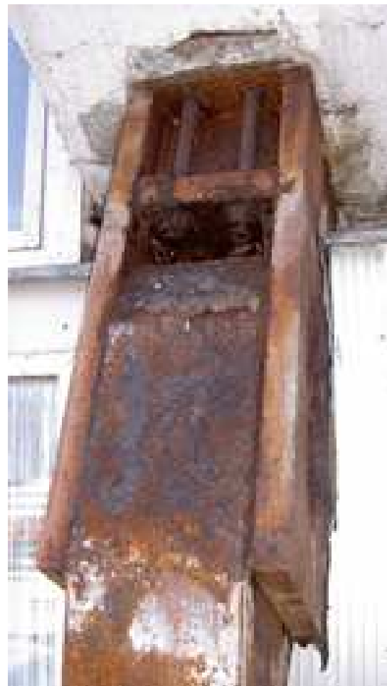
Fig. 4. The corroded joint of the tension rod.
