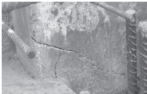
Fig. 5. The view of the object damages resulting from the mistakes in the prestressing process
