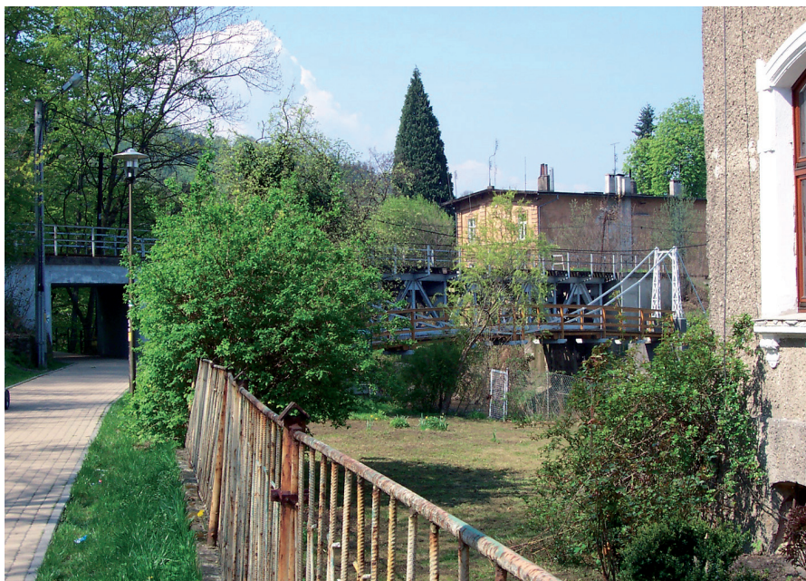
Railway bridge on Biała Głuchołaska among the town buildings – View from northeast
