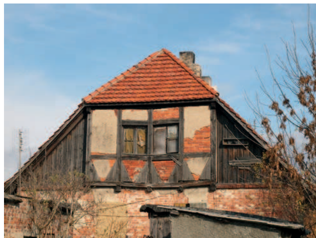
Fig. 2. Granecznik, examples of damage caused by a lack of current repairs and maintenance of wood
