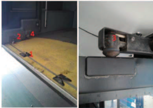
Figure 3. Components of the door system: 1-bottom track, 2-bottom guide, 3-door hinge with a potentiometer, 4-door arm tip
