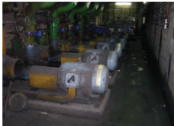
Fig. 7. Pump room where the machine is located
