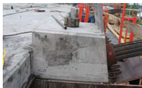
Fig. 3. Damaged cantilever no. 4 after prestressing
