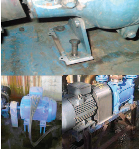
Fig. 5. Rotating machines with a weak bench
