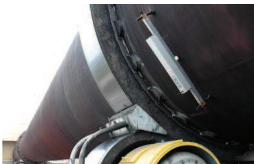
Fig. 9. Shelltester mounted on the rotary kiln's shell
