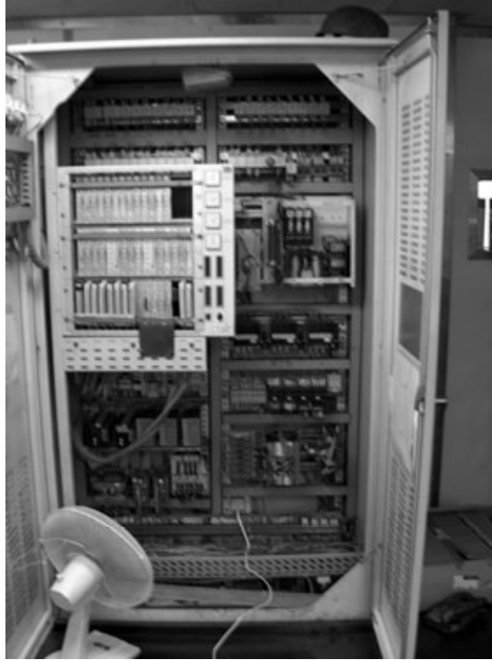
Fig. 1. A view of an electrical cubicle with set of contactors in engine control room
