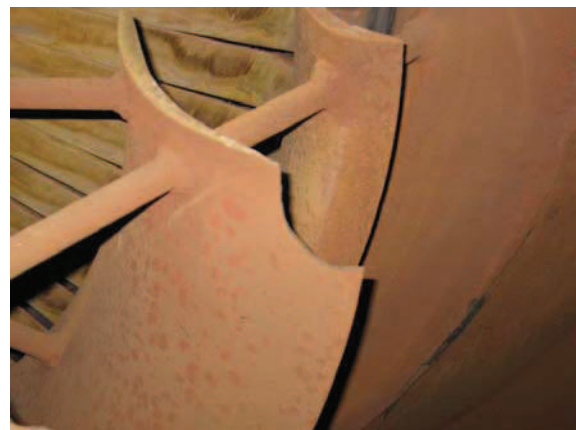
Fig. 5. Photographs of damaged guide fences; in the upper photo, arrows indicate loose welded joints (1) and the guide fence that has fallen off (2); lower photo shows damaged guide fence edge
