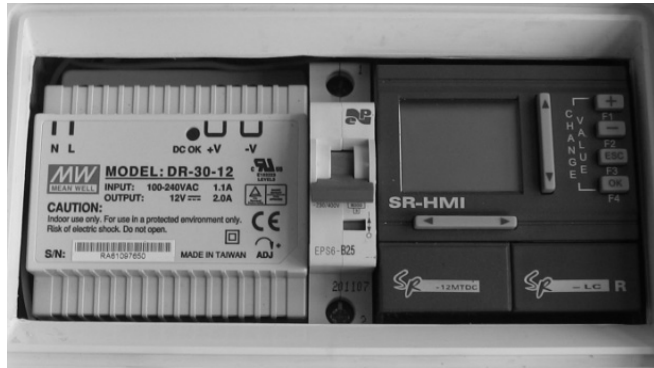
Fig. 3. Front panel of PLC controller
