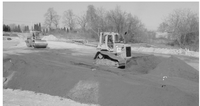
Fig. 5 Construction of ring road of city of Chrzanow using the aggregate-binder blend from Sobieski Mining Company
