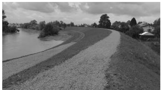
Fig. 6 The construction of dikes alongside the Vistula river using the „dried” aggregate with ash from Janina Mining Company
