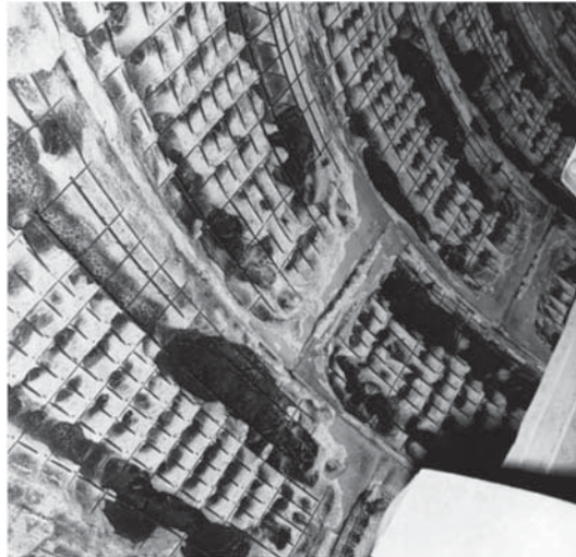
Fig. 2. Damaged structure after the fire in Eurotunnel in 1996 [2]
