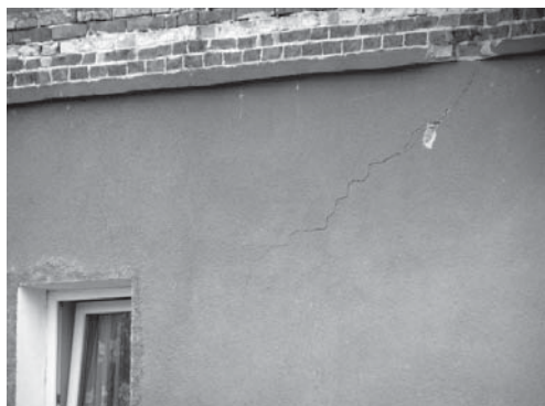
Fig. 14. Cracked walls a single-family building, Kamienna street, which is a consequence of the colluvial masses movement. (Photo by A. Borecka)
