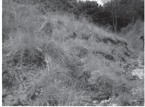
Fig. 9. The crown of the landslide with fresh detachment faults in its northern part, near Lutowka water-course, which shows that there is a very dynamic slip of colluvial masses in the area. There are visible water seepages from the crown of the landslide. (Photo by A. Borecka)
