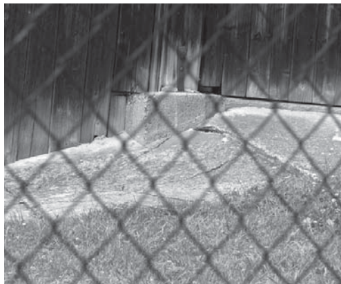
Fig. 12. Cracked concrete pavement near a utility building, Kamienna street, which is a consequence of the colluvial masses movement. (Photo by A. Borecka)
