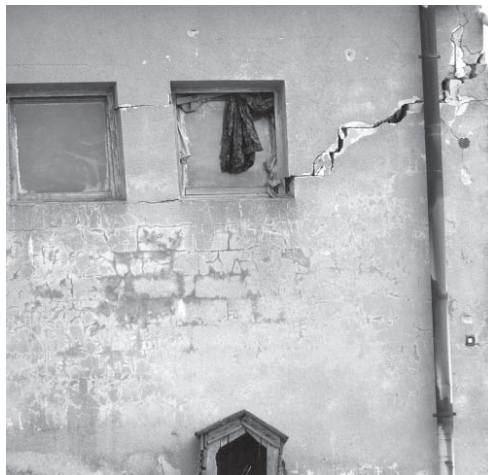
Fig. 13. Cracked walls a utility building, Kamienna street, which is a consequence of the colluvial masses movement. (Photo by A. Borecka)
