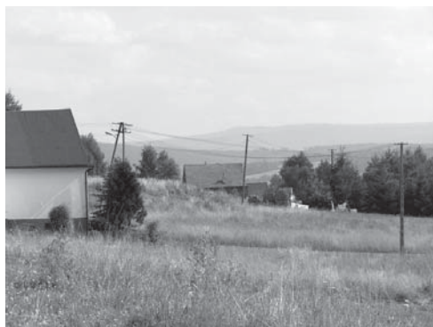
Fig. 15. Tilted pylons near Kamienna street, which is a consequence of the colluvial masses movement. (Photo by A. Borecka)
