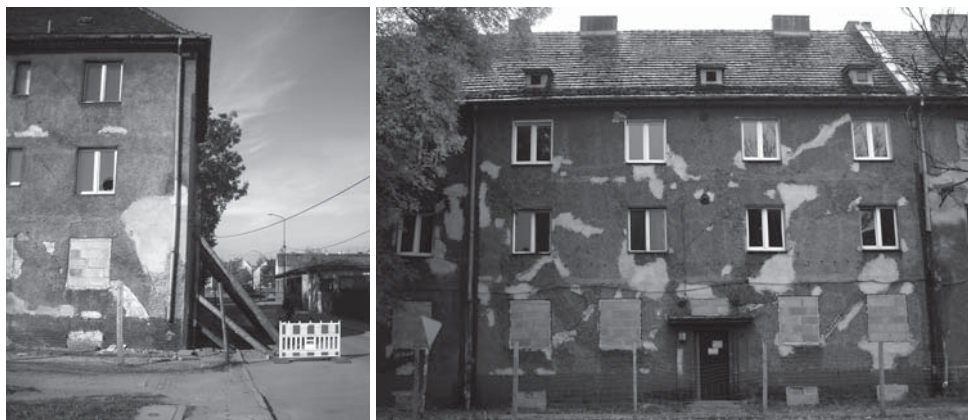
Fig. 2. The loss serviceability characteristics of a structure with the threat to safety state (Bytom Bobrek, 2011, own photos)
