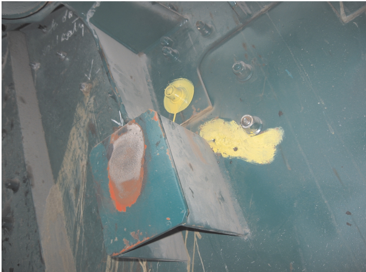
Fig. 2. Fractures in the regions of the sieve sideboard support, damaged HuckBolt bolts
