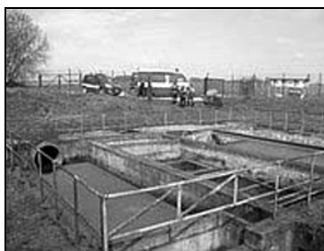
Fig. 2. Lapol D — leaks of oil products
